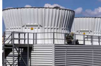
Cooling Water Treatment
