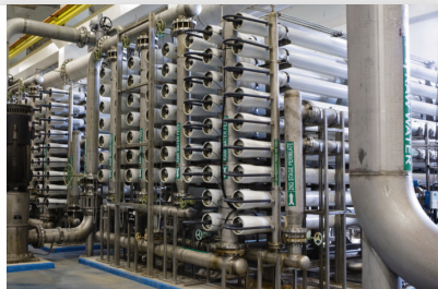
RO Membrane Treatment
